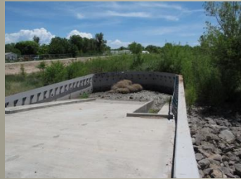
Sanchez Farm Inlet (trash/sediment removal structure)
