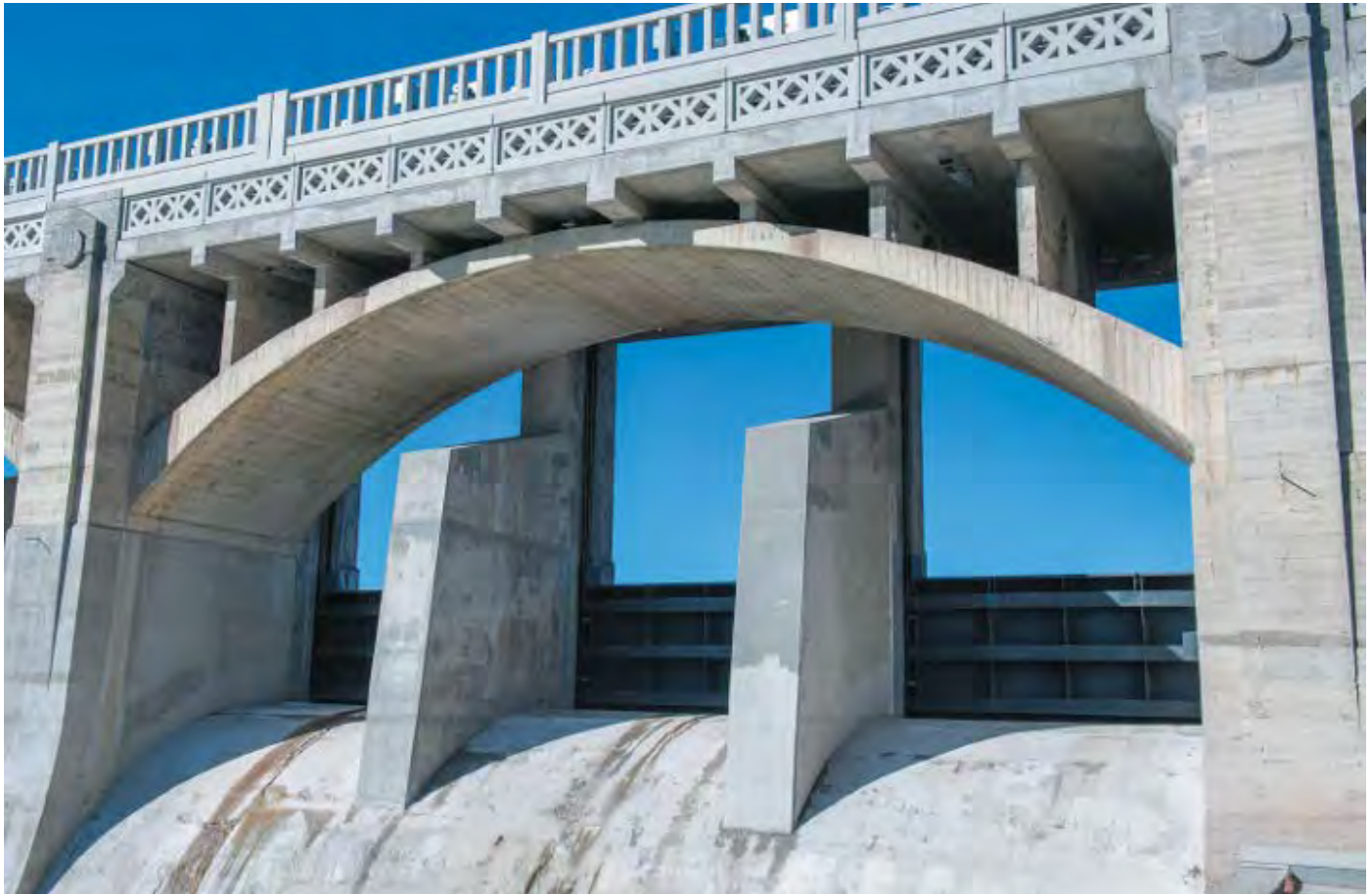
Newly installed steel gates at the Glenmore Dam provide an extra 10 billion liters in storage for greater flood protection along the Elbow River. As winter approaches and flows along the Elbow River slow, the gates allow the City to store double the amount of water in the reservoir, which helps meet the needs of a growing city. Source:
